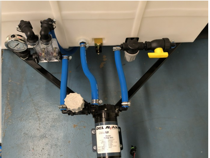
Figure 10: Main plumbing Assembly
